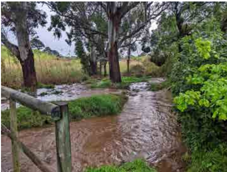
Figure 17: The path to the Tokai greenbelt is repeatedly flooded and has been extensively damaged, and the water course is increasingly widening. Note the levels of sediment in the river. The river has widened to encroach on private property to the right of the photo.
